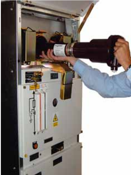
Fusarc CF fuses installed in a CAS 36 cubicle
